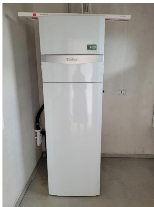
Hot water tank
