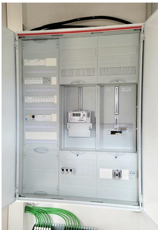
Meter main distribution
