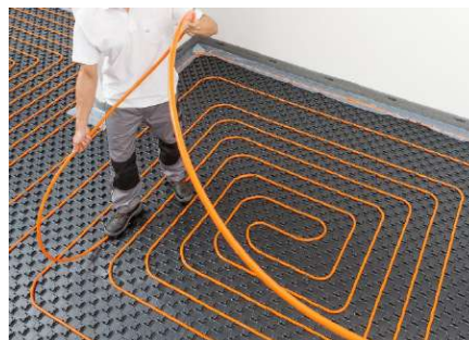
Hot water under-floor heating
