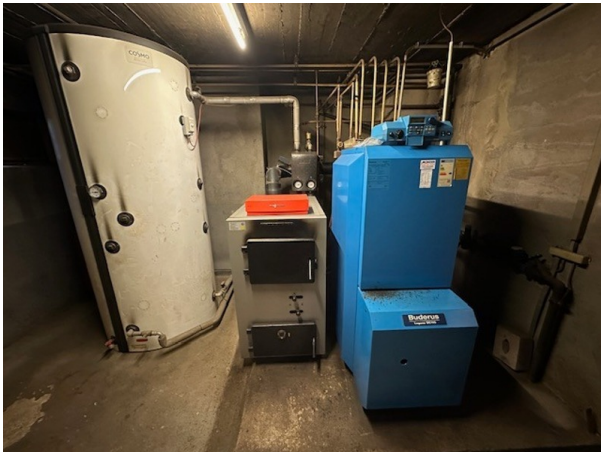
18_KG_Heizung Holz BJ2014 + Öl BJ2004
